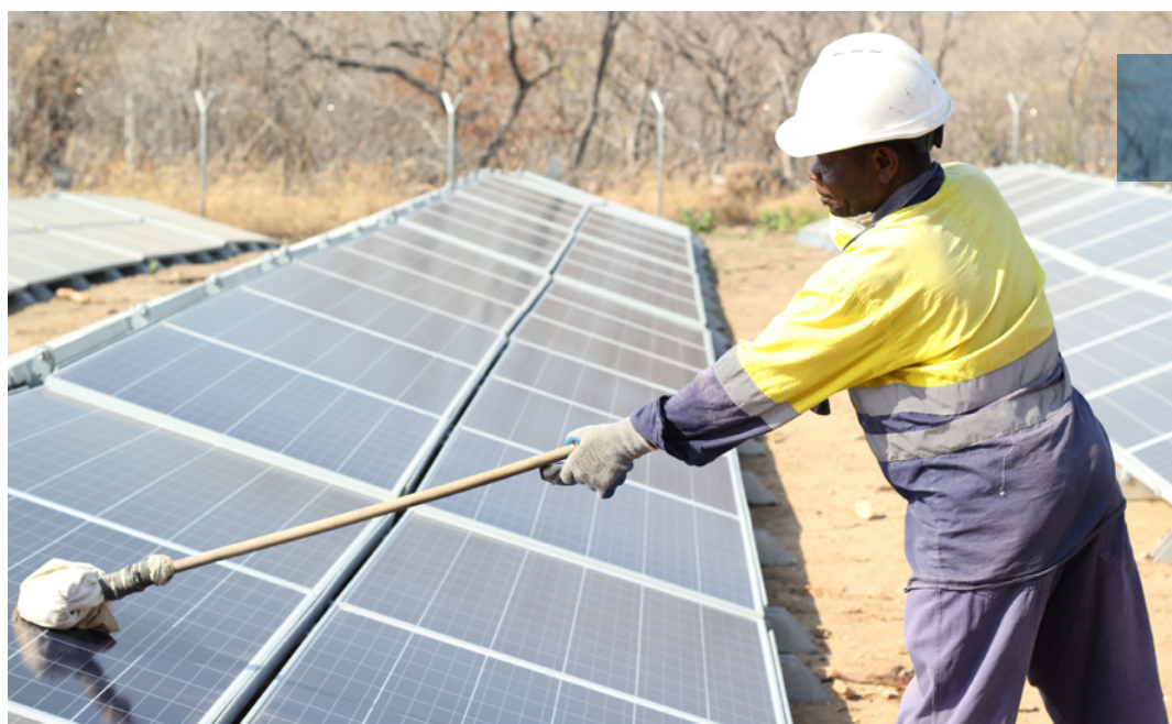
Man cleaning solar panels
